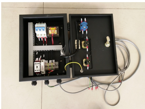
Fig 1: GB control box with additional wires
